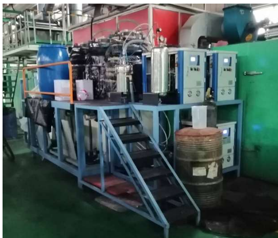
Complete storage and feeding tanks units
